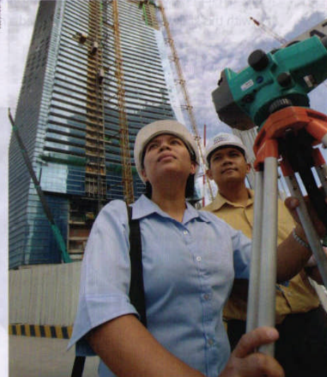
Tritech engineering staff hard at work at the Marina Bay Financial Centre
